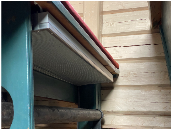
(a) Pew-mounted Heating Panels
