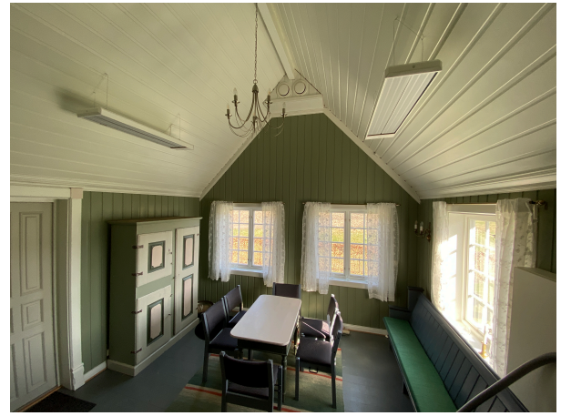
(b) Heating Panels Hanging from Ceiling, 1700W
