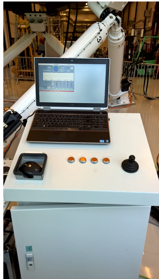
(b) Control cabinet and HMI during testing
