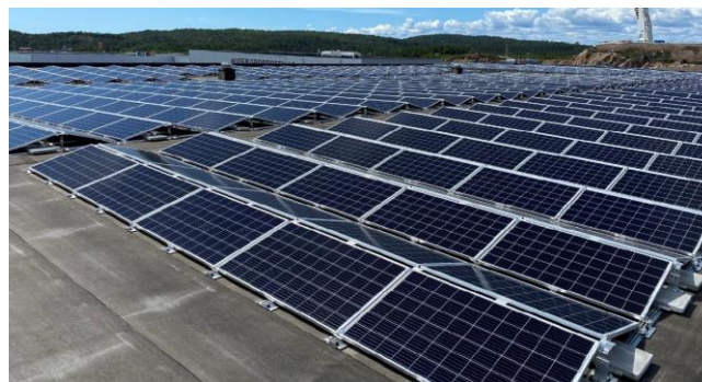
Figure 26. Gorines' roof equipped with solar cells.
