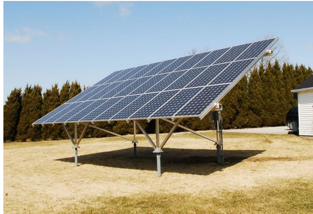
Figure 3.8 : Solar PV ground mounted system [29].
