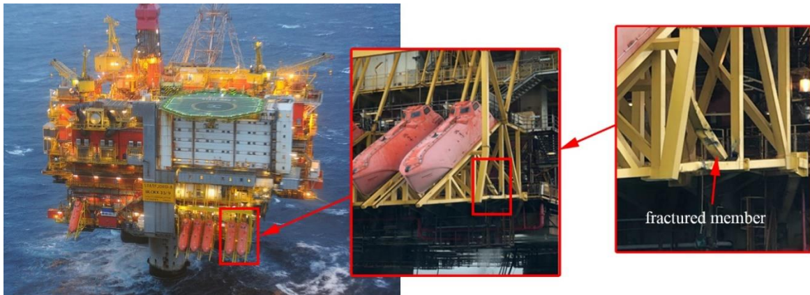
Figure 1.8. Sjøborg supply vessel collided with the Statfjord A platform and caused damage to the lifeboat structure in 2019 [59, 66].
