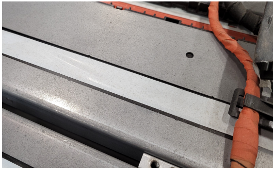
(a) White tape placed along battery modules.
