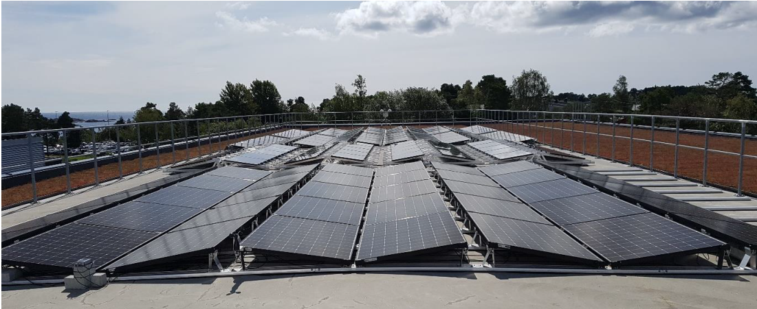
Figure 7: The PV system situated on the roof of UIA campus Grimstad
