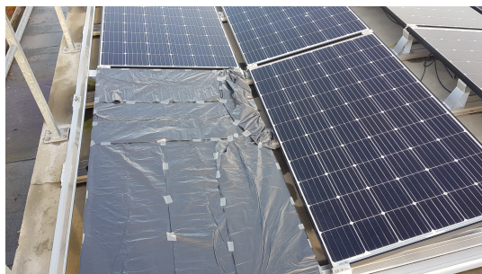
Figure 13: Module K4 is completely covered
