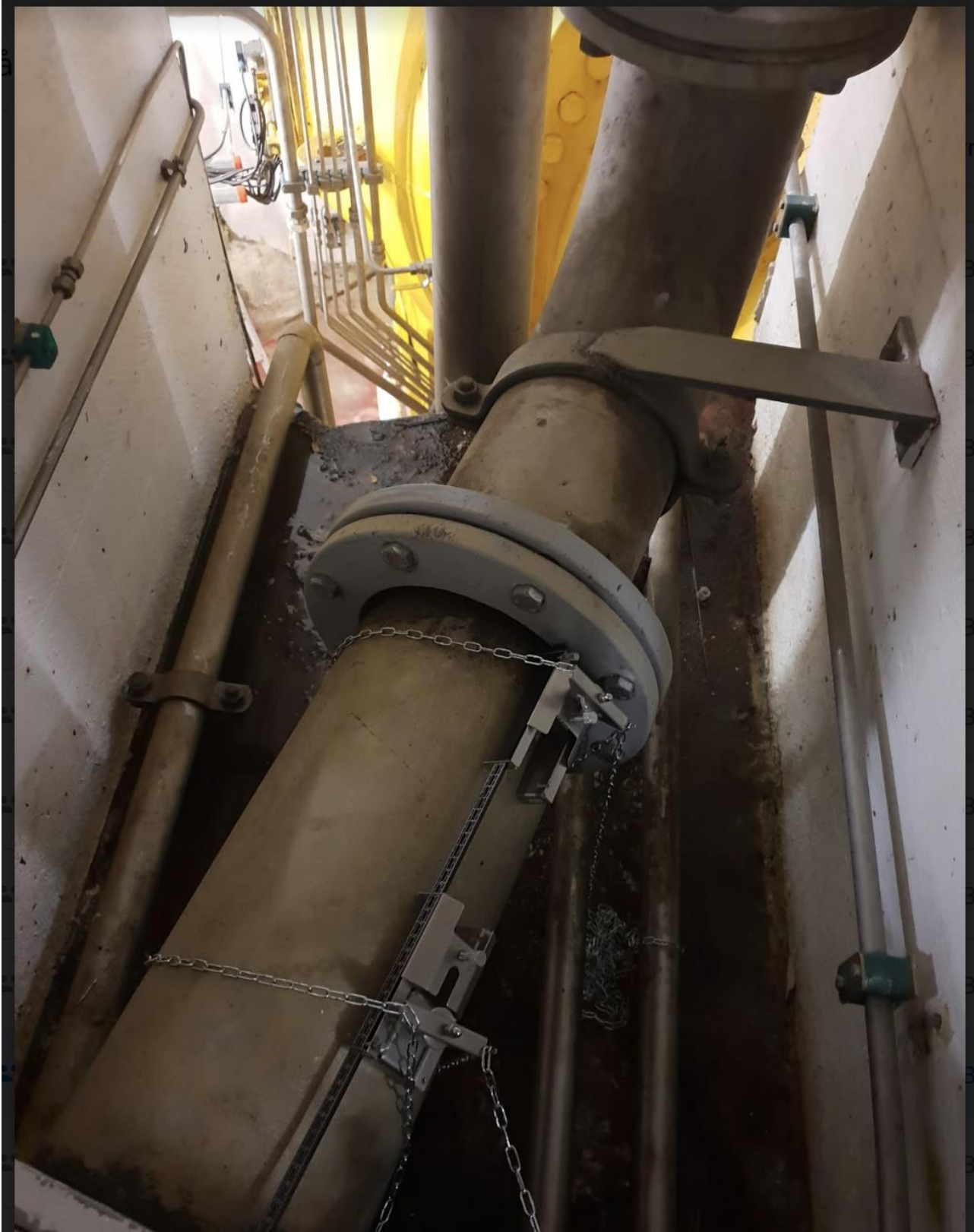
Figure 66: Measuring point 1 PF220B at Brokke.
