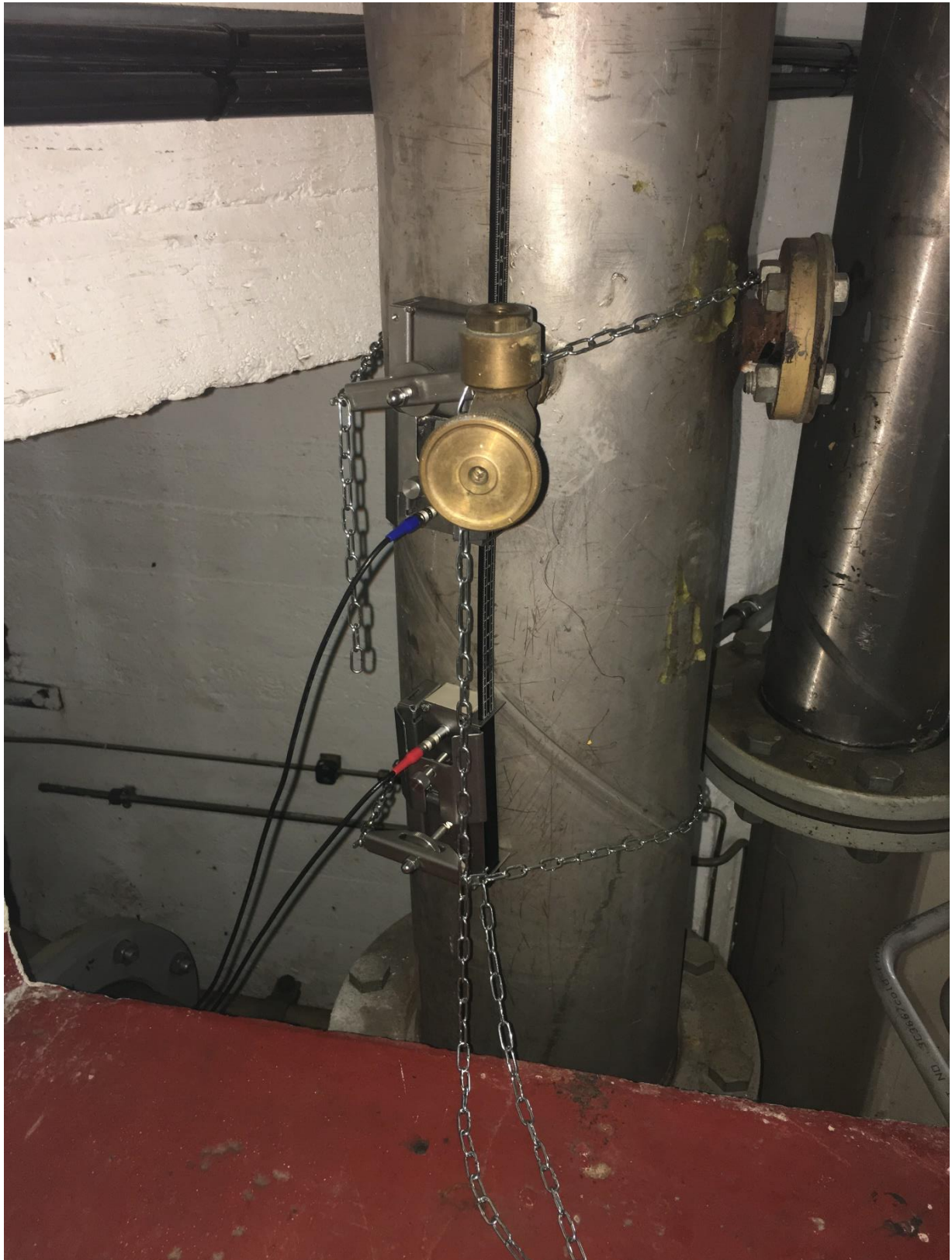
Figure 67: Measuring point 2 PF220B at Brokke.
