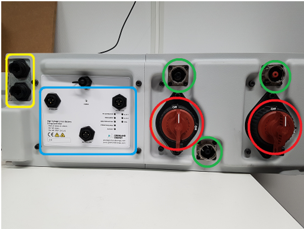
Figure 3.27: Marked EE-Top switches and plugs
