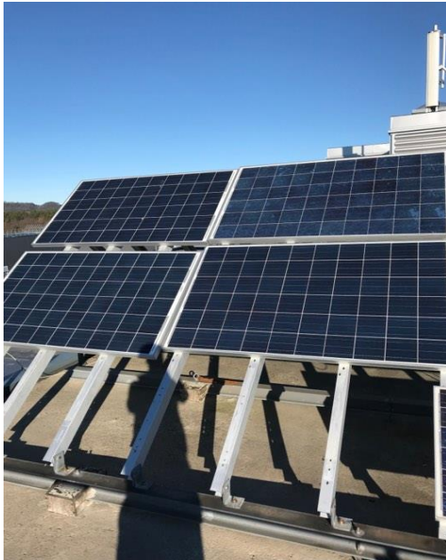
Figure 23 Picture of the 4 PV panels used.
