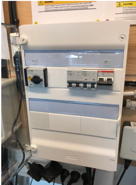
Figure 27 Fuse box in the PV lab.
