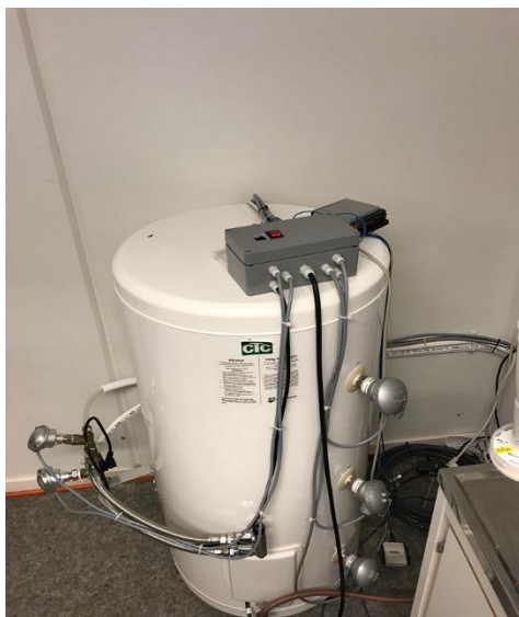
Figure 35 Hot water tank with junction box and thyristor at top of it.
