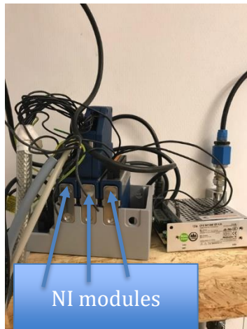
Figure 28 Overview of the NI modules connected to the hot water heater and labview.
