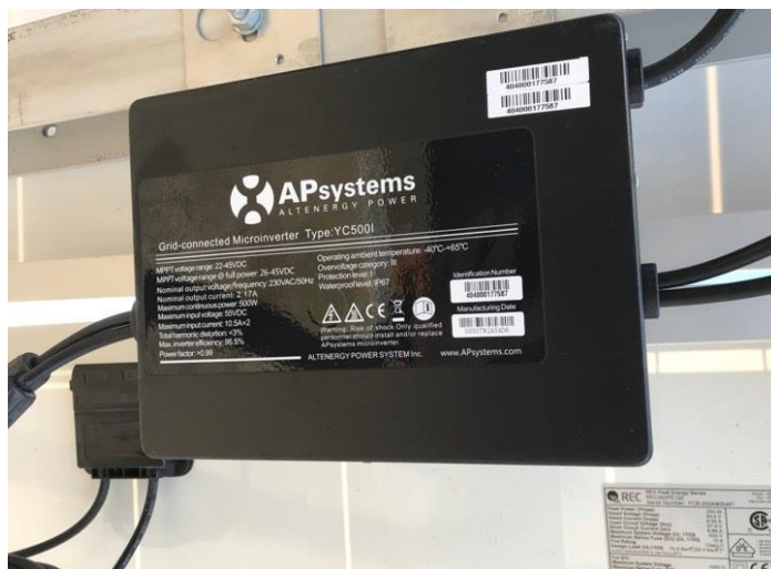
Figure 26 Micro grid inverter mounted at back on the PV panel.
