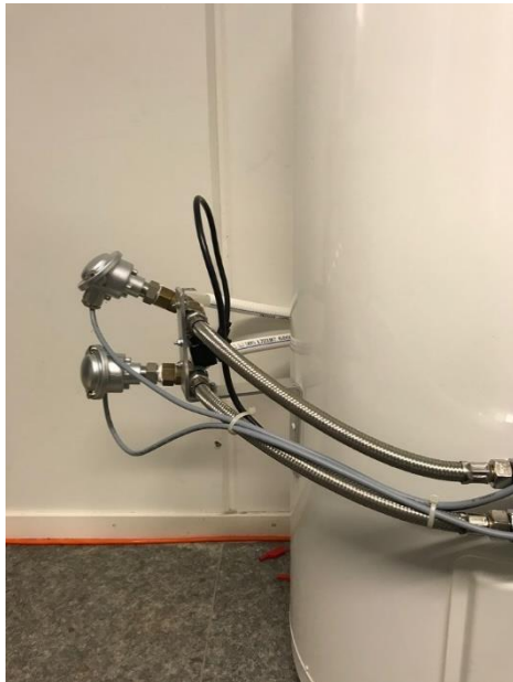
Figure 29 In this picture the valve controller for the water tank is shown.
