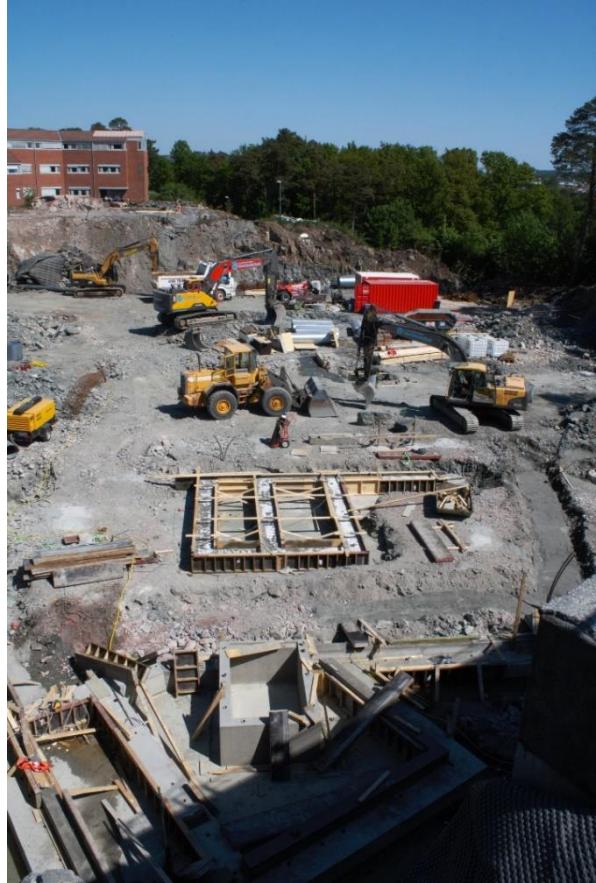
Figure 1 Basic work for the construction of the new health lab at the University of Agder (self-taken photo, 24th of May 2018)
