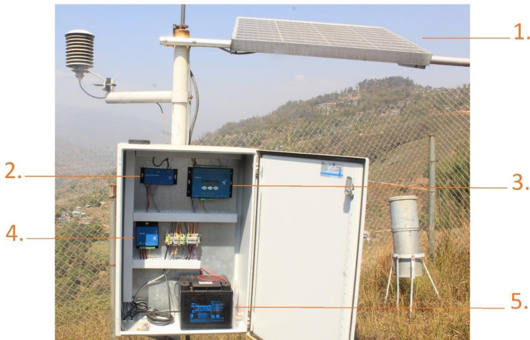
Figure 4.2: Automated Rainfall Station for the EWS Installed in Ilam
