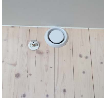
Figur 6.17. Tilluftsventil i stue
