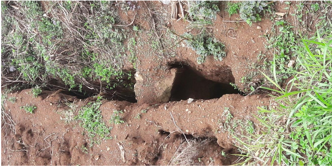
Figure 10: A crack identified by community members is Bunabutiti parish
