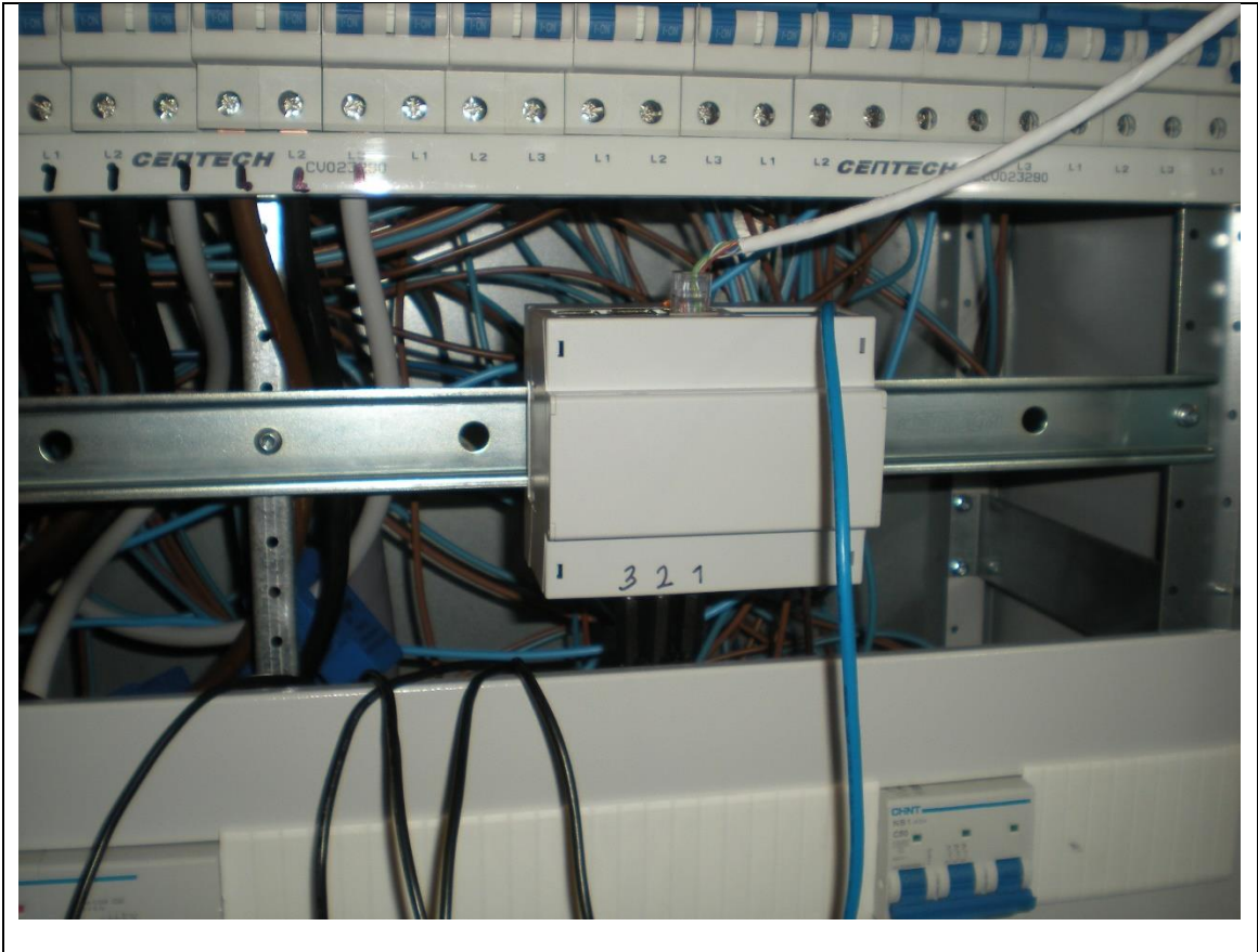
Figure 3-27 Raspberry mounted on DIN rail in a fuse box
