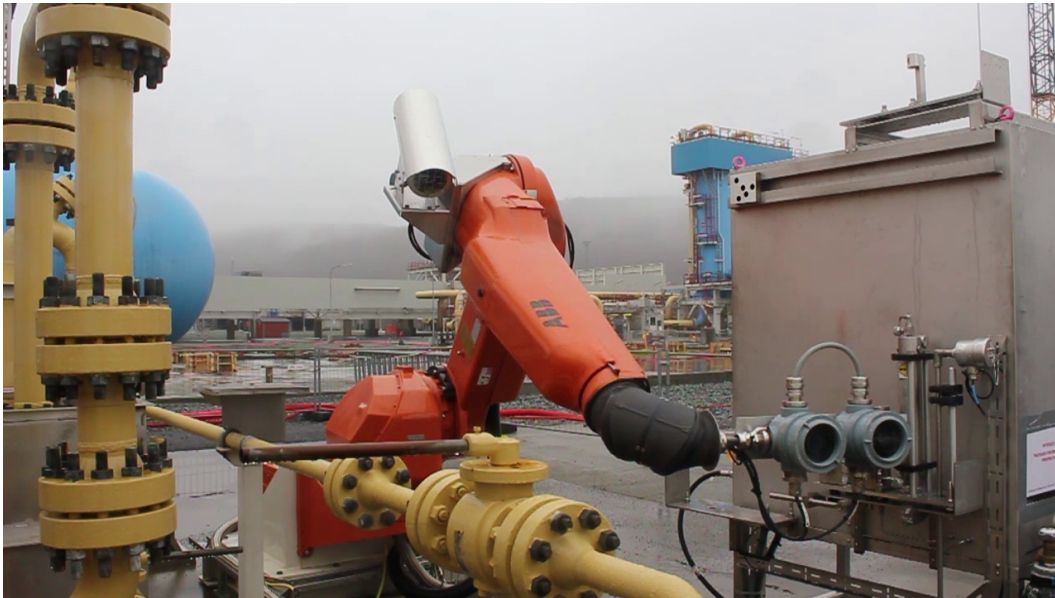
Figure D.2: A robot located in a potentially explosive environment, among pipes carrying gas. This shows a state of the art petrochemical related application for industrial robots.
