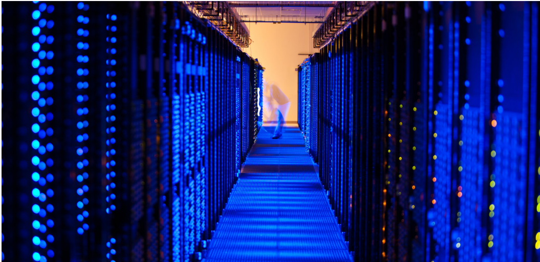
Figure 2.8: Computers facilitating massive parallel computing at Amazon’s web services data centre. (Photo courtesy of The New York Times)
