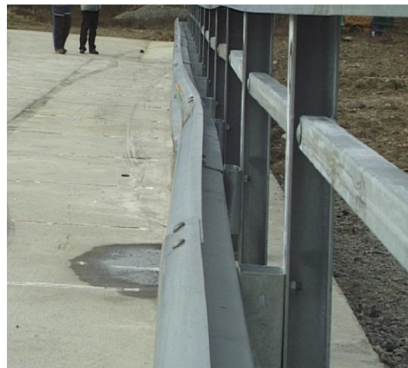
Figure 17. Safety barrier – location of impact.
