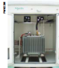
Transformer in PV box
