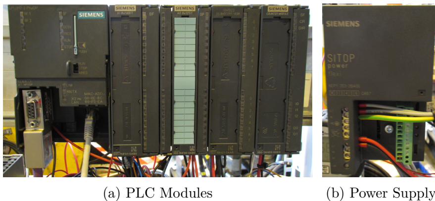
Figure 7.4: Siemens S7 modular PLC
