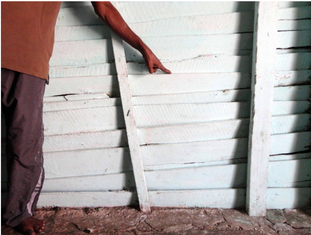
Photo C: Demonstrating the water level inside the house during floods. Source: Author
