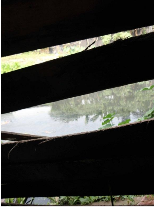
Photo A: The channel behind the shack is visible through the cracks in the kitchen wall; a breeding area for mosquitos and other insects. Source: Author
