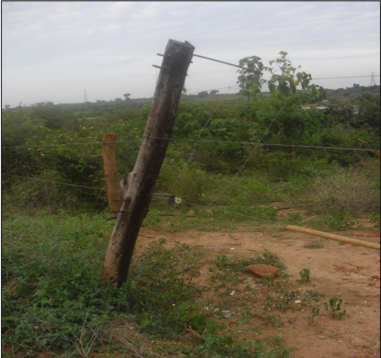
Figure 18: (Photograph by Researcher) Deteriorated pillar
