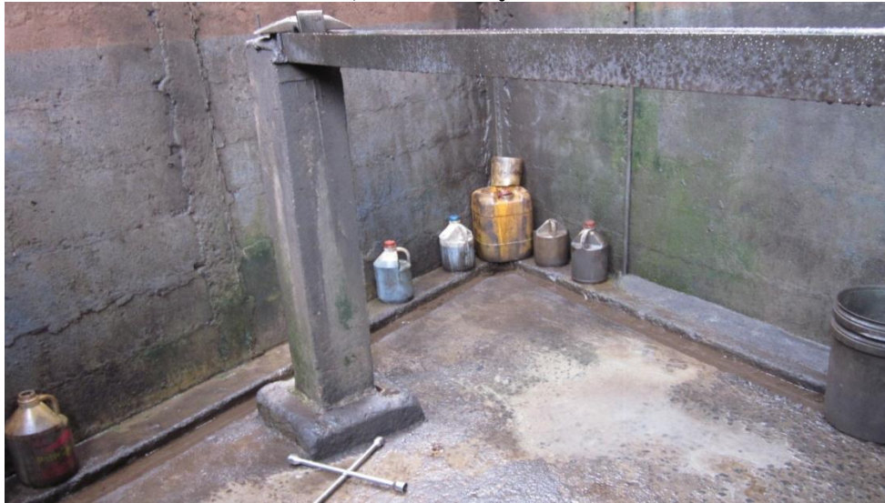
Photo 10: Unsafe work floor, not friendly to the environment
