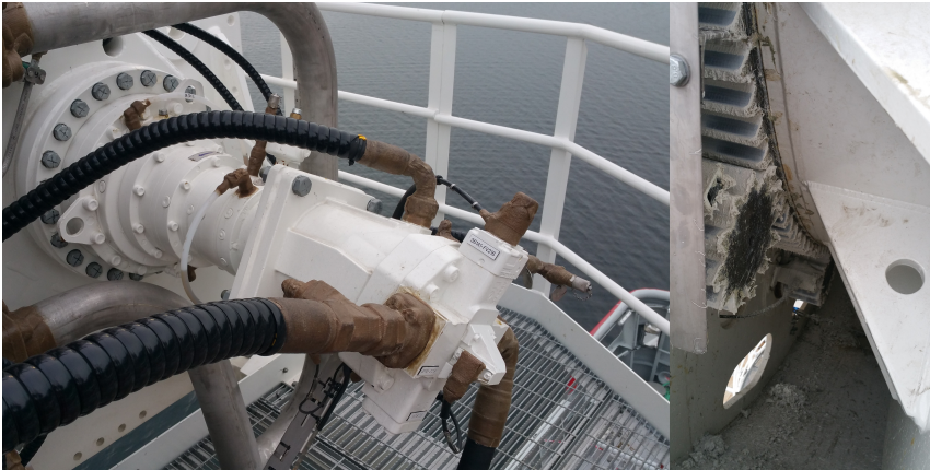
Figure 2.10: Motor and pinion system on L4593
