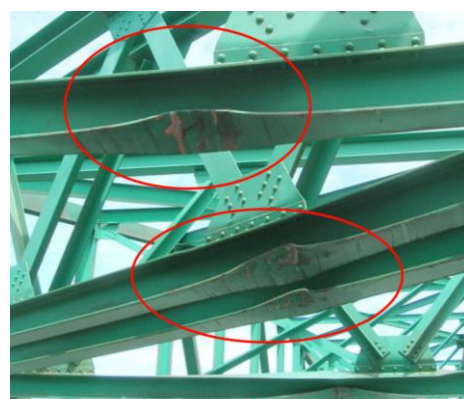
Figure 6 Damage to trusses caused by collision [50]
