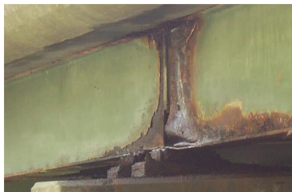
Figure 5 Rusted steel beam under a bridge [48]
