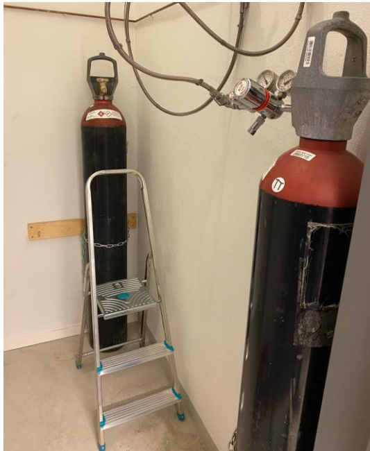
Figure 19 Tanks containing hydrogen
