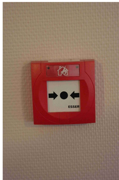
Fig. 3 Fire alarm call point in the living room of an apartment
