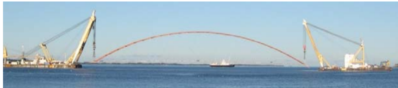
Figure 16. The 220m span of the Brandanger Bridge, moved to the pillars by big floating cranes.
