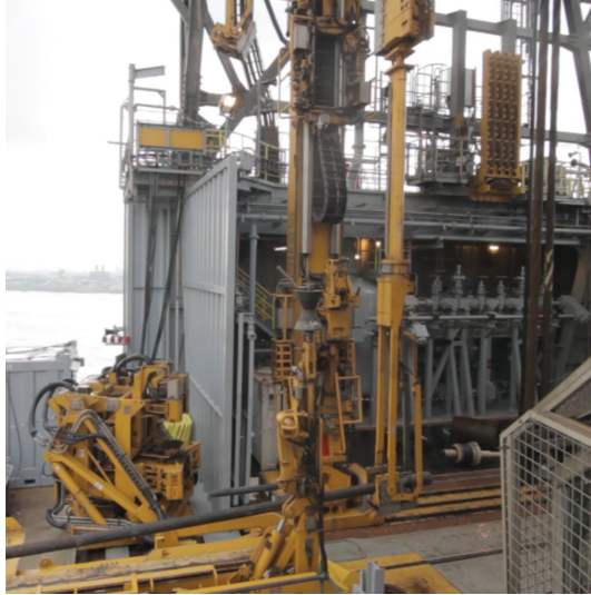
Figure 2. Modern pipe handling using Multi Machine Control (MMC) from NOV. The operator visually confirms the pipe hand-over position between robots before resuming automatic sequence. See full video at go.nov.com . (Image, NOV.)
