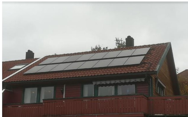
Figure 5 Housed equipped with solar panels supplied from Solcellekraft AS
