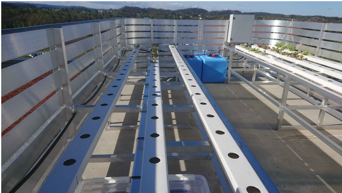
Figure 4.7: Rooftop system with two water containers and six tubes
