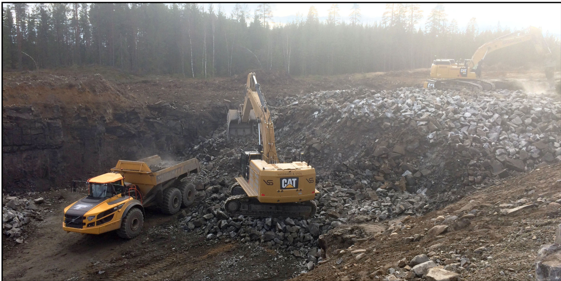
Figure 5.2: Photo taken at the case. The image shows one of Skanska's Volvo articulated trucks working together with a Cat excavator from Vassbakk & Stol [56].
