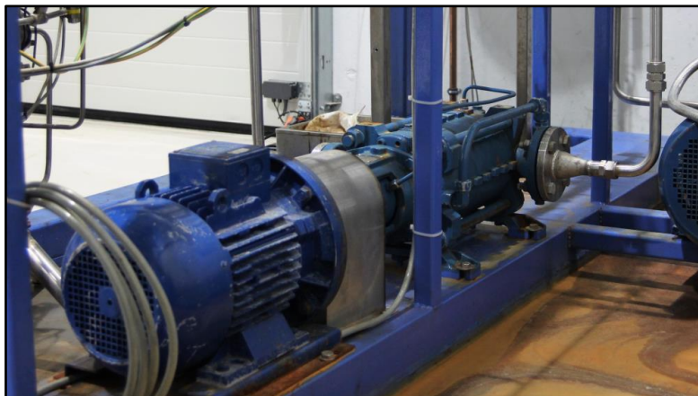
Figure 4.6: Picture of the coalescing multistage centrifugal pump.
