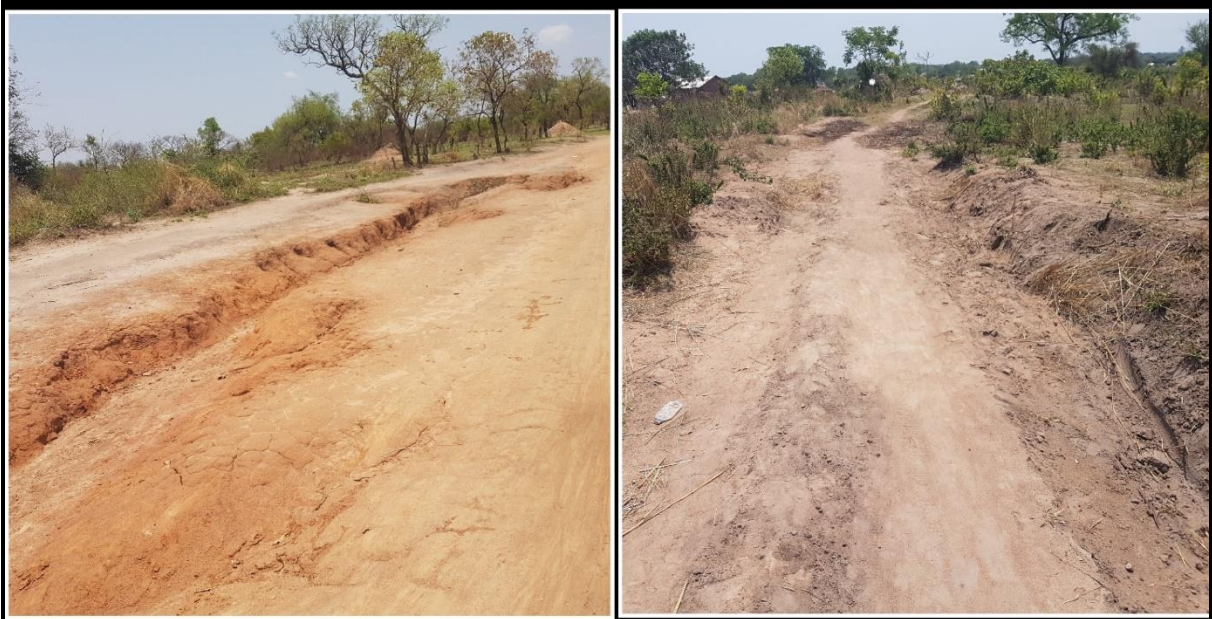
The state of the access roads in the settlement, on this they look better because it is in the dry season. Photo: Tererai Obey Sithole.
