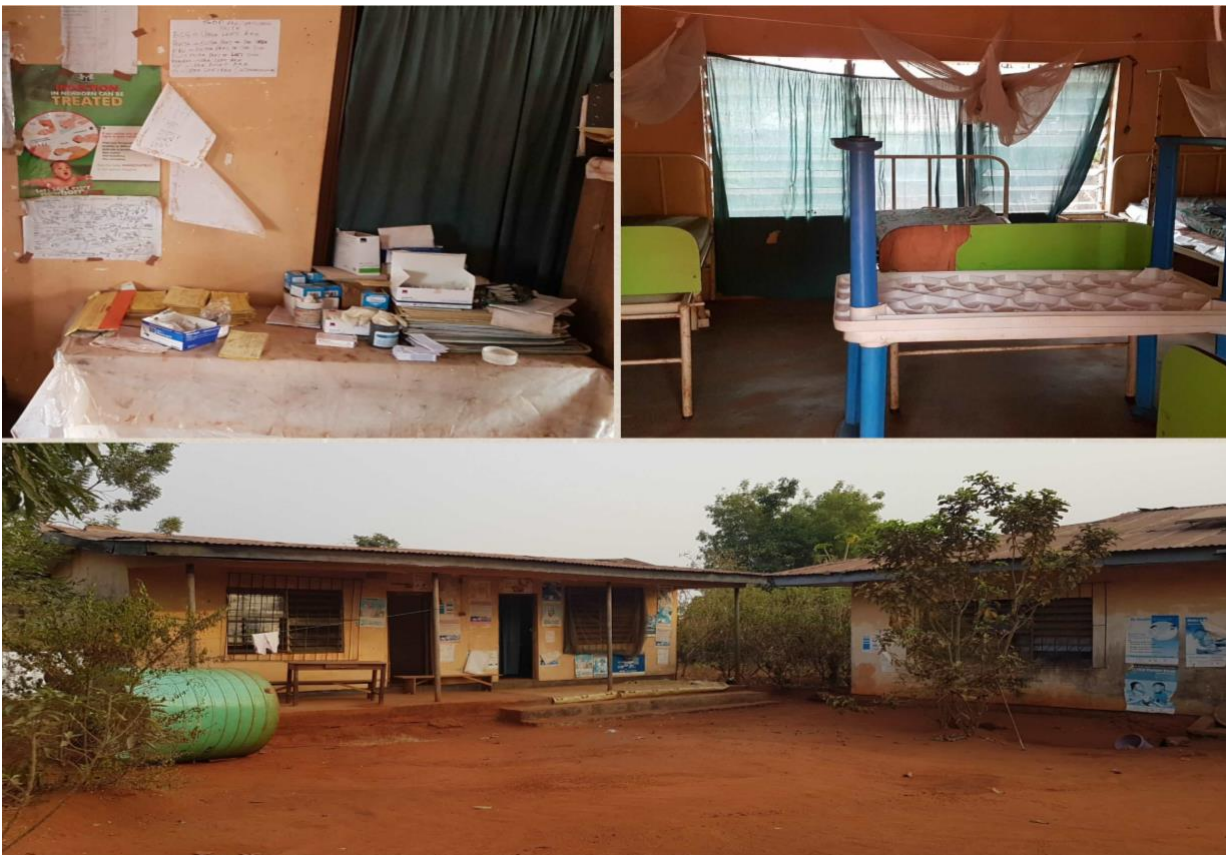
Picture 4: Poor condition of primary health centre (PHC) in Nando and Aguleri community
