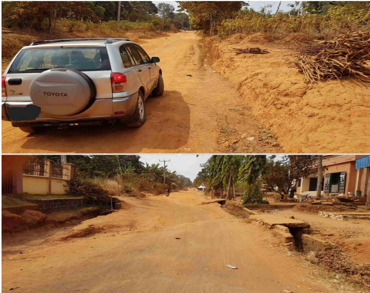
Picture 1: Uncompleted road construction and bad roads in Nando and Aguleri community.
