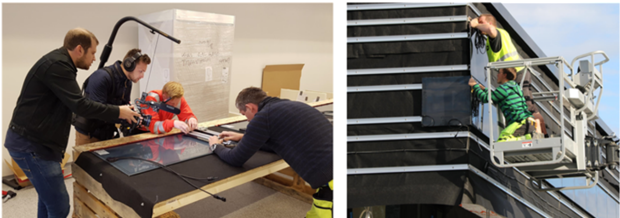
Figure 5.28: Gluing and installation of the PV modules at Kiwi Dalgård, retrieved from [74]
