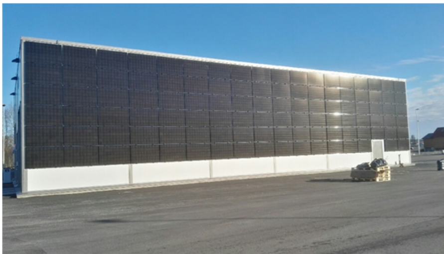
Figure 5.36: The BAPV system on the facade of ASKO washing hall located in Vestby
