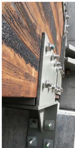
Figure 11 Larger steel parts trapping moisture
