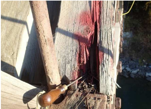
Fig. 9 Fungal Decay in a Diagonal
