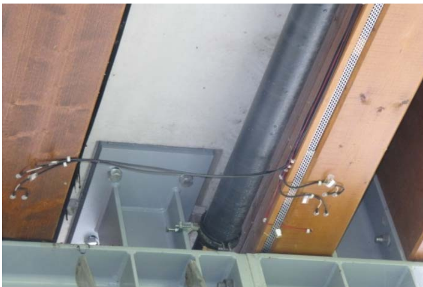
Fig. 5: Two measuring areas above the river at the bridge deck (left) and the tie beam (right)
