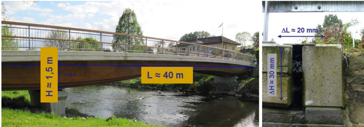
Fig. 5 Advanced and double axis elongation at larger timber bridges results in special demand for expansion joints
