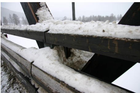
Figure 3 Dense snow being thrown onto the structure by snow blowing equipment
