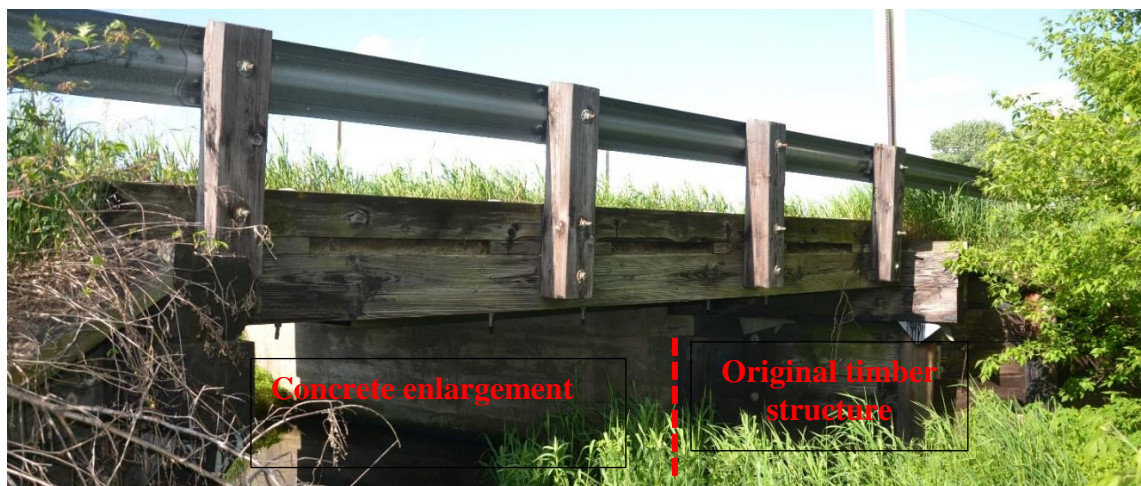
Fig. 4 Timber bridge enlarged with concrete members that has been wrongly codified as a TCC bridge
