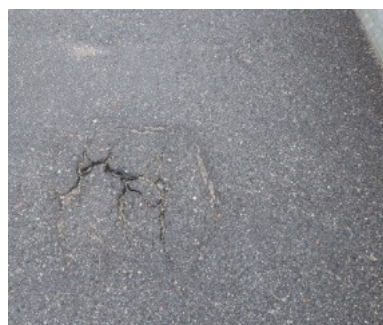
Fig. 3 Blistering of asphalt surface
