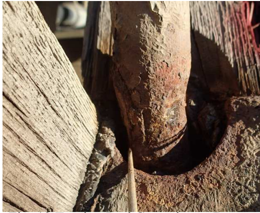
Fig. 12 Tension Rod Corrosion at Base
