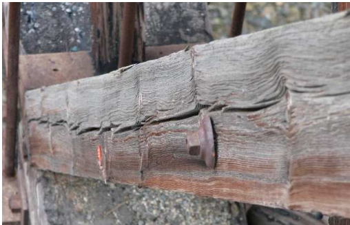
Fig. 10 Weathering and Checking in a Diagonal With a Noticeable Bow
