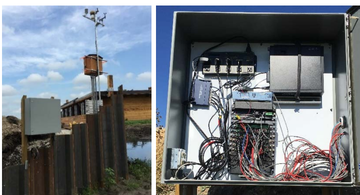
Fig. 7 GRS-Timber Bridge data logger enclosure
