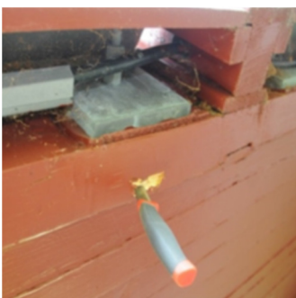
Fig. 2 Moisture damage, decay in outer beams
