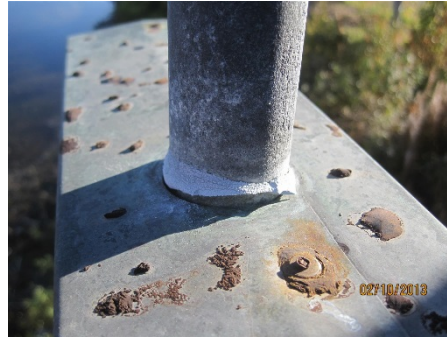
Figure 13 Hangers connected to cladding with broken sealant
