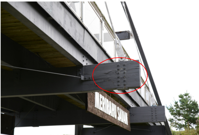
Fungal damage of the transversal beam
