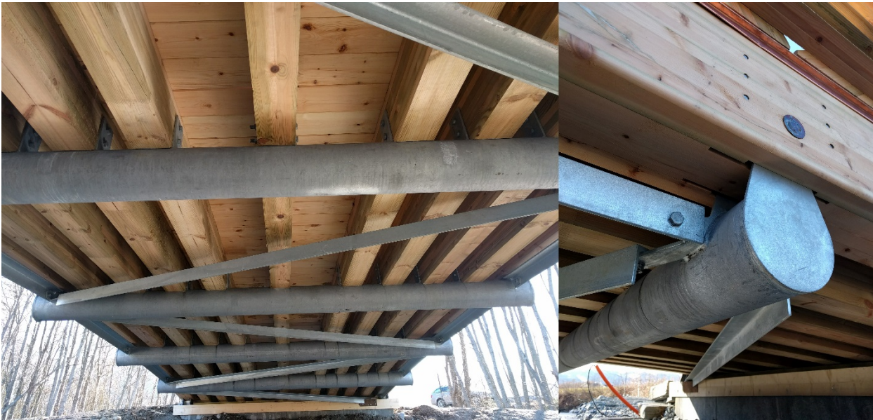
Figure 4: Structural principle seen from below. Picture on the right shows the bottom chord node and the steel truss connection
