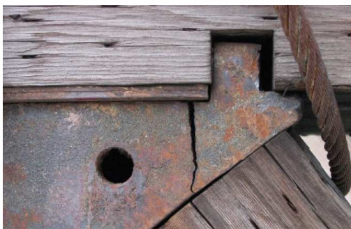
Fig. 11 Cracking in a Top Angle Block
