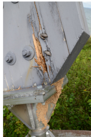
Rotten zone and insects in the arch foot
