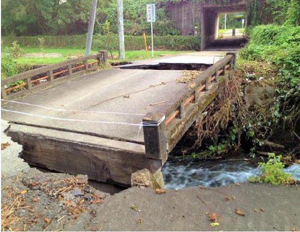
Fig. 1 Broken road bridge
