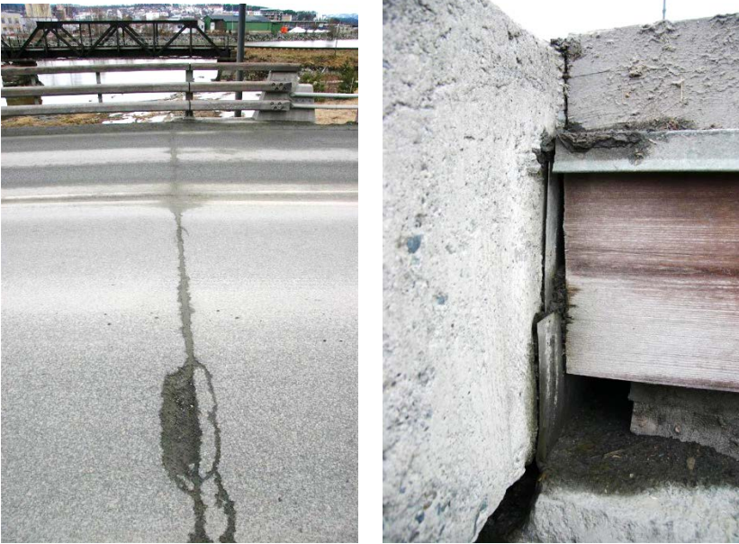
Figure 17 At the transition between timber and concrete, rotation of the deck creates a gutter that leads water towards the end grain of the deck. Over time, dirt is gathered and moisture levels are heightened.
