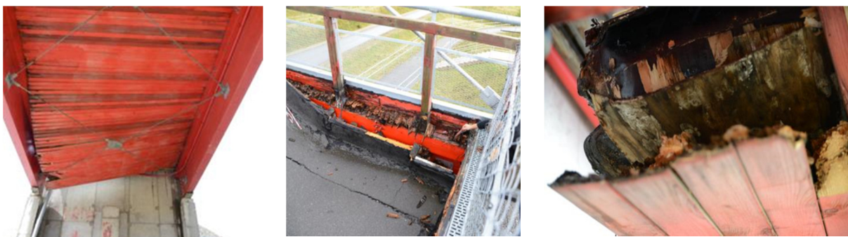
Fig 5. Collapse of the deck in 2014 due to completely rotten deck at supports.
