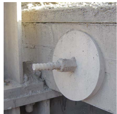
Figure 6 Dirt on the side of the deck on onto the cross beam in direct contact with the deck. Note also that the wood is crushed beneath the anchorage plate also leading to higher moisture levels.
