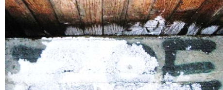
Figure 5 Rime (white) on the underside of a deck close to a cold abutment
