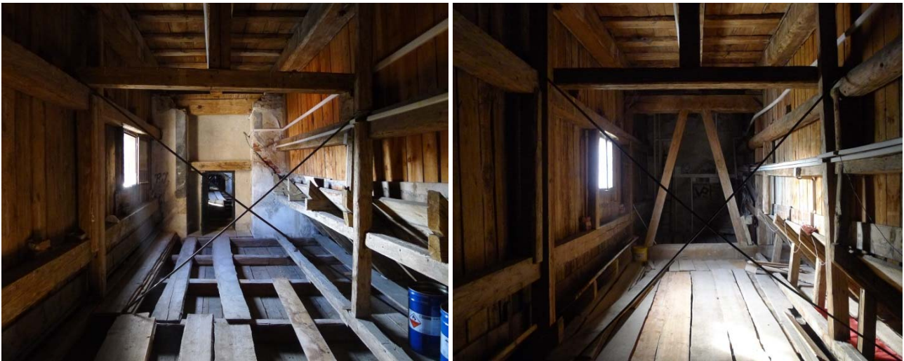
Fig. 5 The space inside the technical storey is divided into three sections, each one illuminated by a single window. In the most westerly section the transversal timber frame (in the background of the right picture) was placed above the pair of slender pillars standing on the terrace in front of the theatre building.
