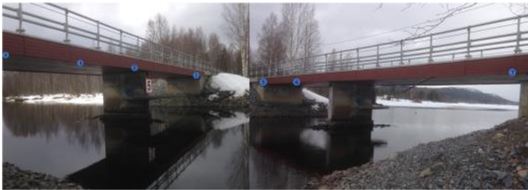
Fig. 8 a, b the sensors marked on a: the north facing side and b: south facing side of Sundbron bridge.
