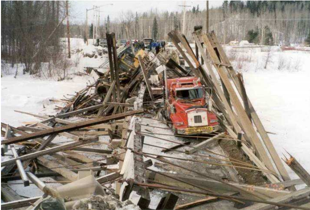
Fig. 4 Collapsed Howe Truss Bridge, Struck By Heavy Equipment on a Crossing Truck
