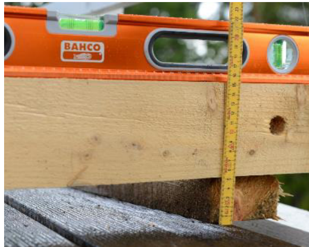
Bridge deck tilted 52mm /m, due to local failure in the arches connection points.
