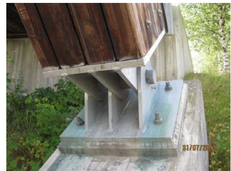
Figure 10 Copper corrosion on hot galvanized steel parts from the cladding
