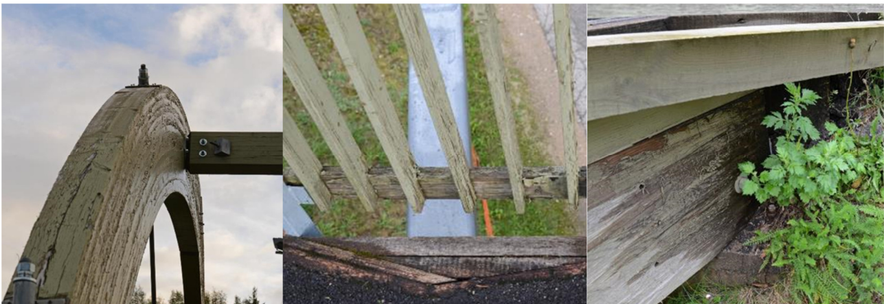
Arches need re-painting and covering on top Railing needs replacement
