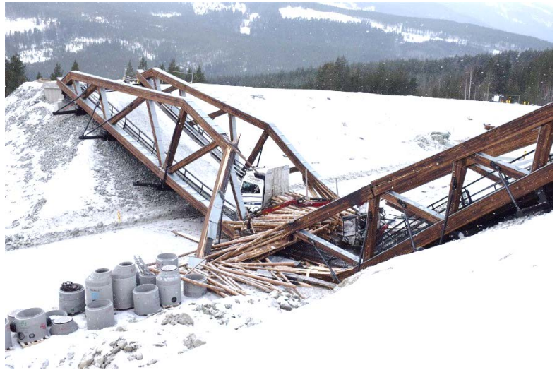
Figure 1 Perkolo Bridge after collapse
