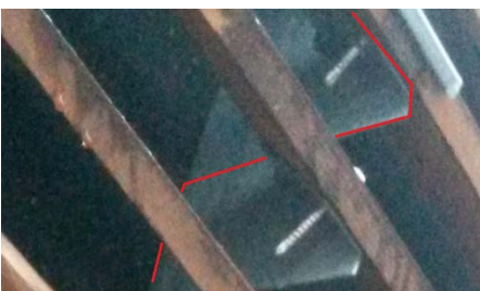
Figure 12 Water runs on the underside of the louvers. If the fixing is beyond the edge of the louvers water may be directed back onto the timber as shown in red line.
