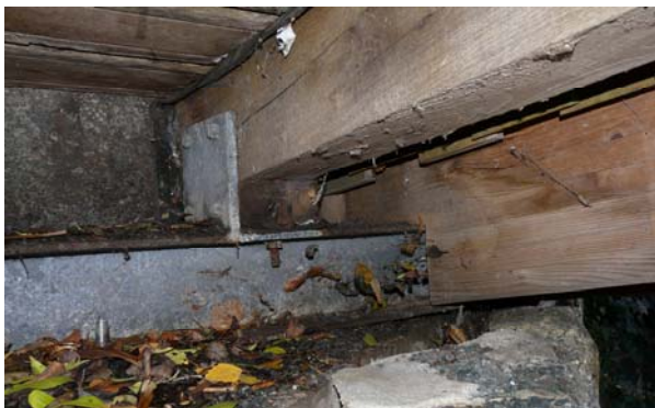
Fig. 3 Closed areas around bearings with dirt, rotting leaves and high humidity
