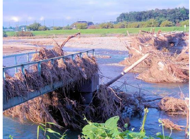
Fig. 2 Broken foot bridge
