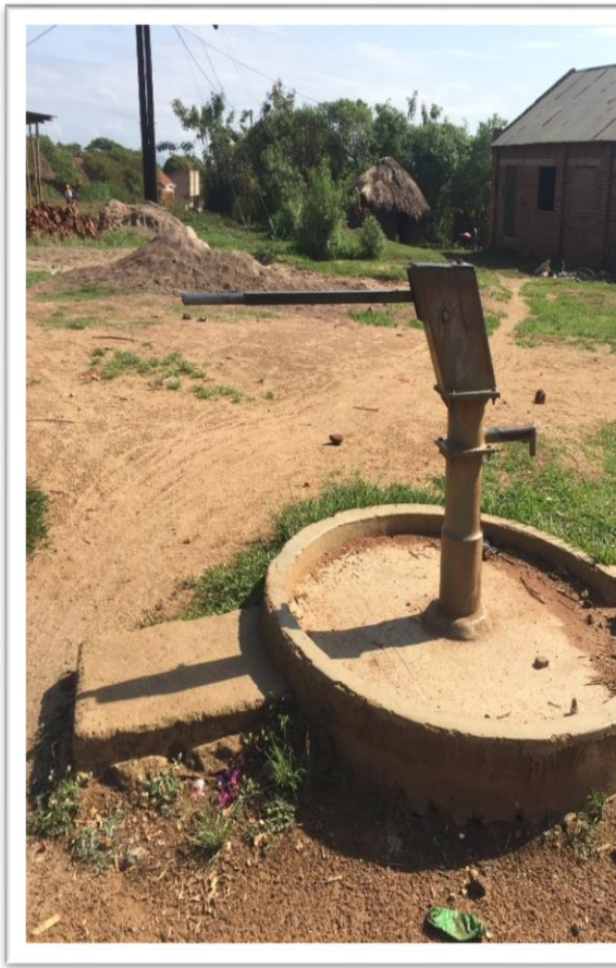
Figure 16: Non-functional Nasinu village borehole
