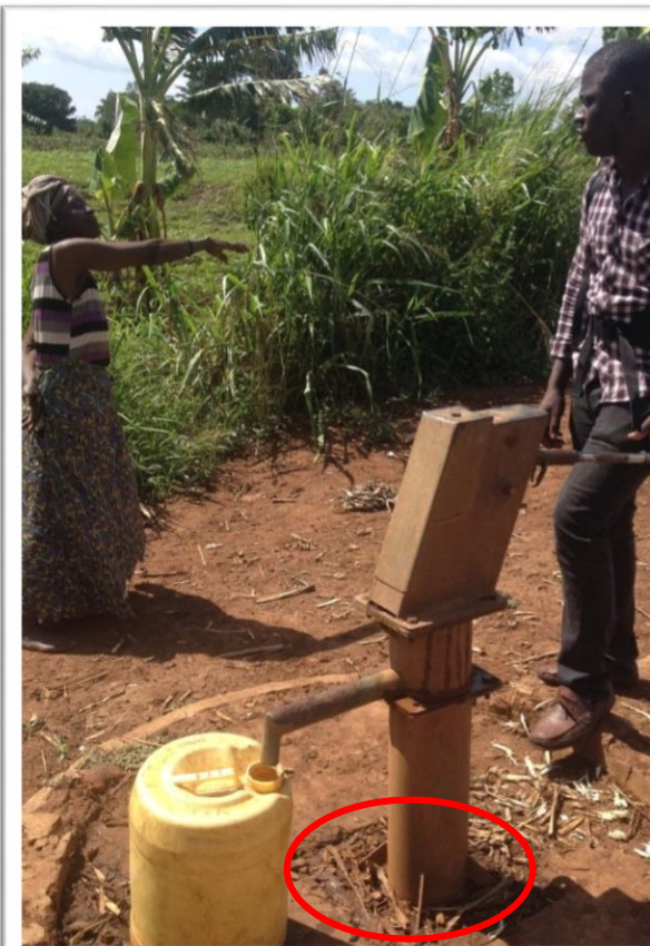
Figure 25: Bukoova shallow well with maintenance issues, under poor sanitation
