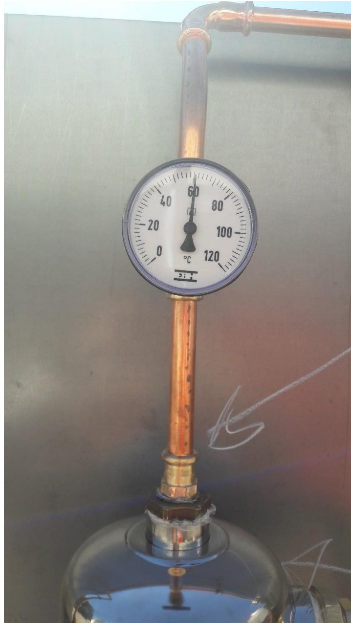
Figure 4-17: The thermometer measuring the temperature of the heating fluid.
