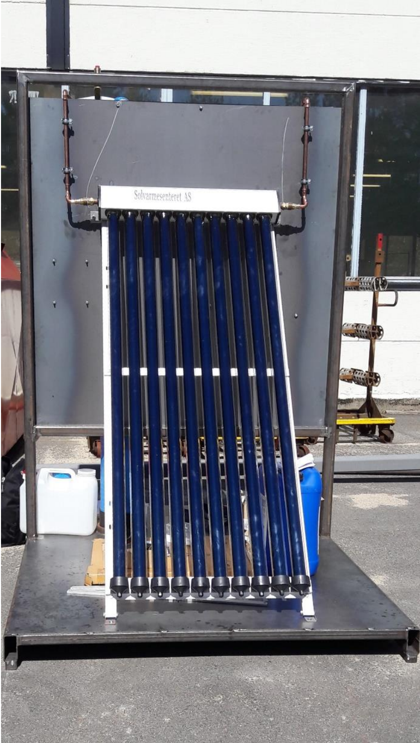
Figure 4-15: The finished system seen from the solar collector side.
