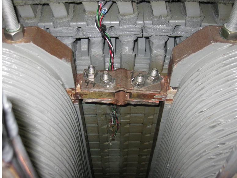
FIGURE 4.9: Cable routing of the upper cables
