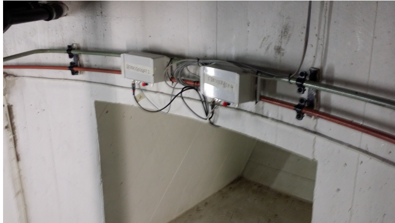
FIGURE 4.13: Connection-boxes ready for measurements in Suldal 1
