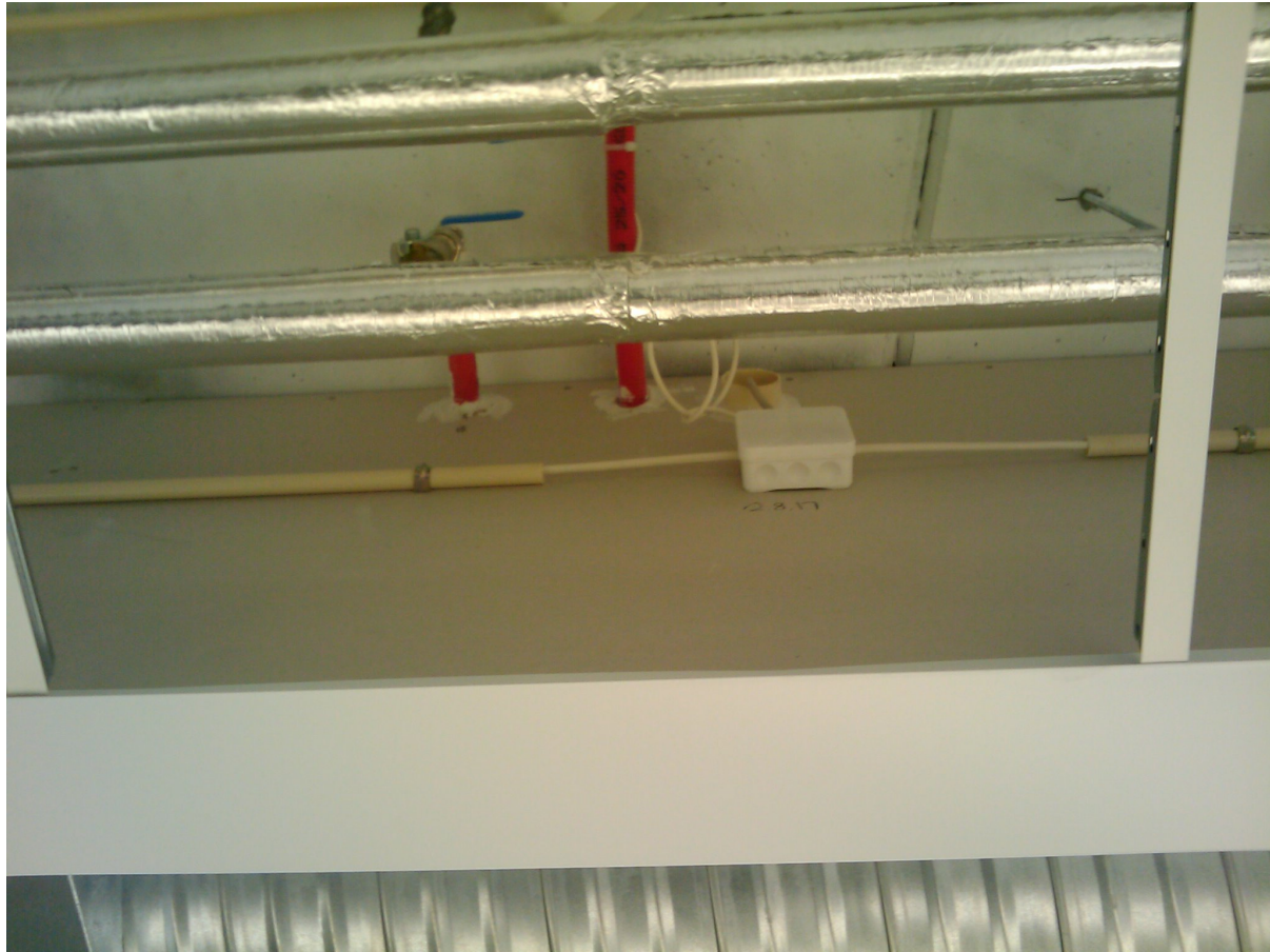
Figure 3.4: An example of work done incorrectly at a construction site
