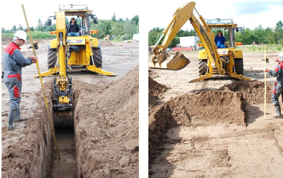
Figure 6: Trenching with 600mm bucket (left) and removal of overburden with an incline leveling bucket (right).
