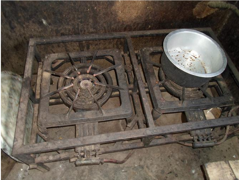
Figure 3.5 Two of the four biogas stoves at Katulani SS
