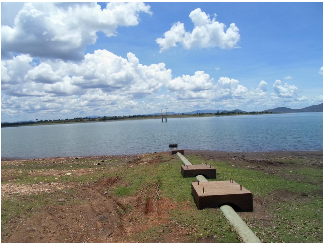
Figure 3.1 Masinga Dam showing submersible pump and pipe line towards Kitui.
