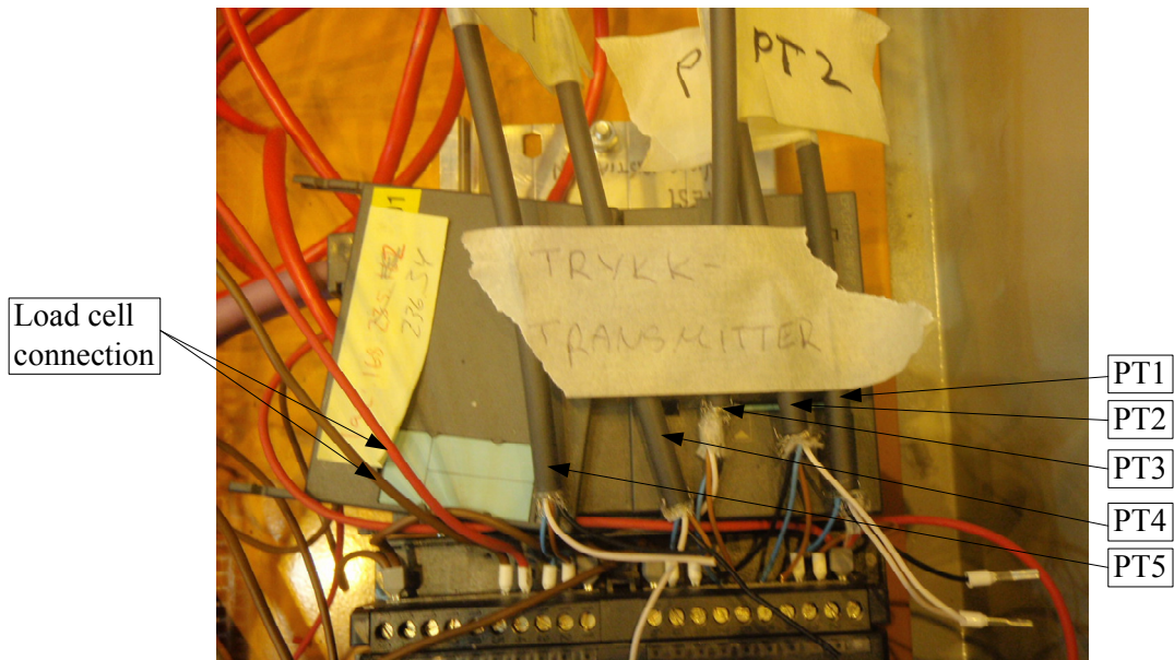
Fig 5.11 Analog input connections from the load cell and the pressure transmitters PT1-PT5
