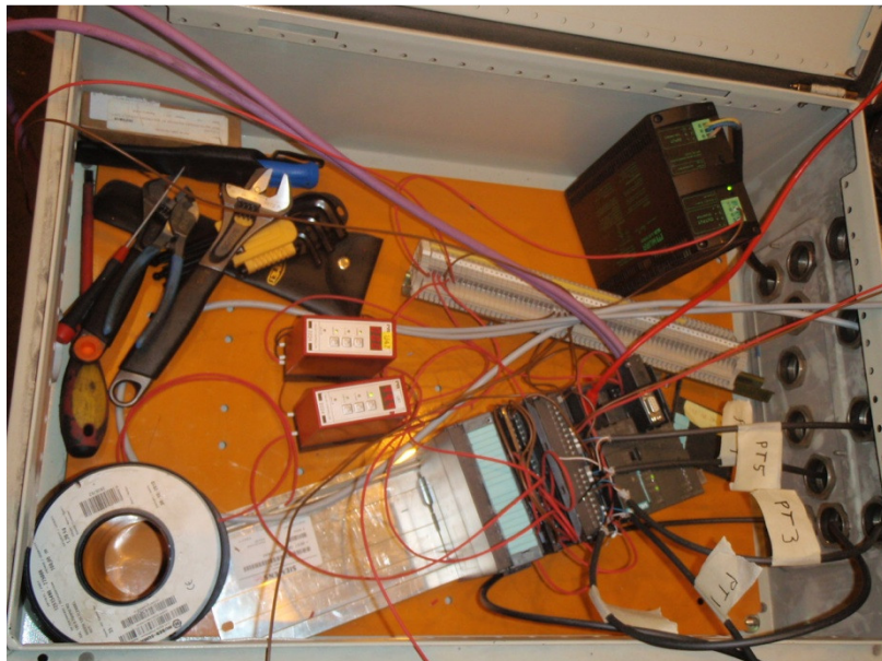
Fig 5.14 Overview picture of electrical system
