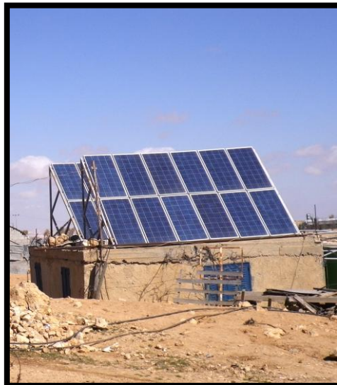
Figure 6.3: Solar Panels in Bedouin Encampment
